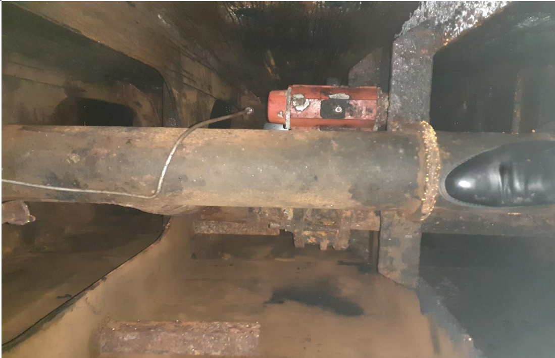
Fig.3. General view of the studs of the ballast pipe (top view)
