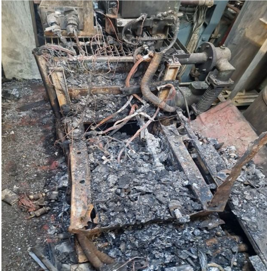
Fig. 4.10. Image of the base of the rectifying group 022
