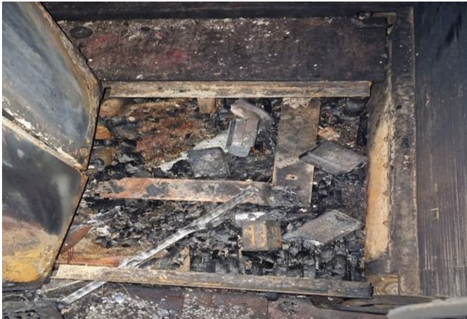
Fig. 4.12. Image of the burst capacitors.
