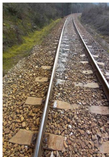
Fig. 2.2. Rail track condition after the rederailment of the 16th wagon
