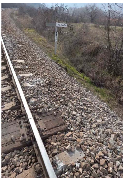
Fig. 2.1. Point of rederailment of 16th wagon
